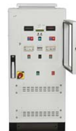
Two power supply units
